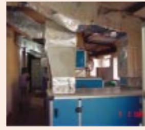
Air Handling Unit
