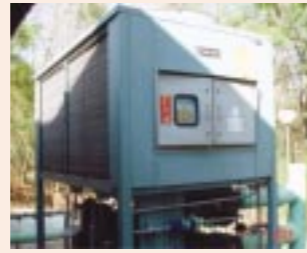
Air Conditioning Unit
