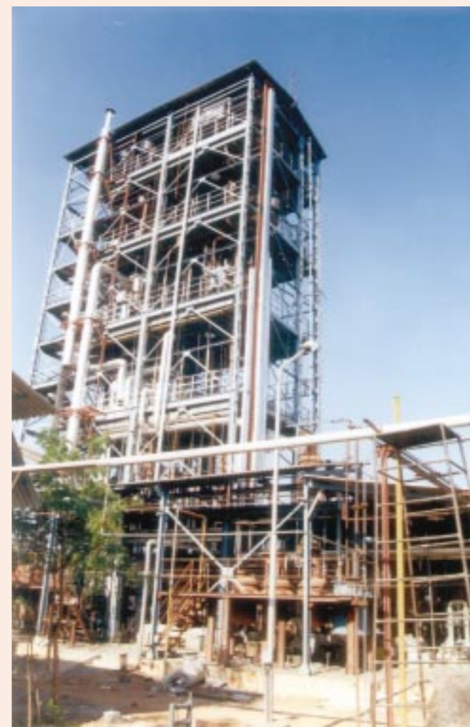
HFC 134a Pilot Plant
