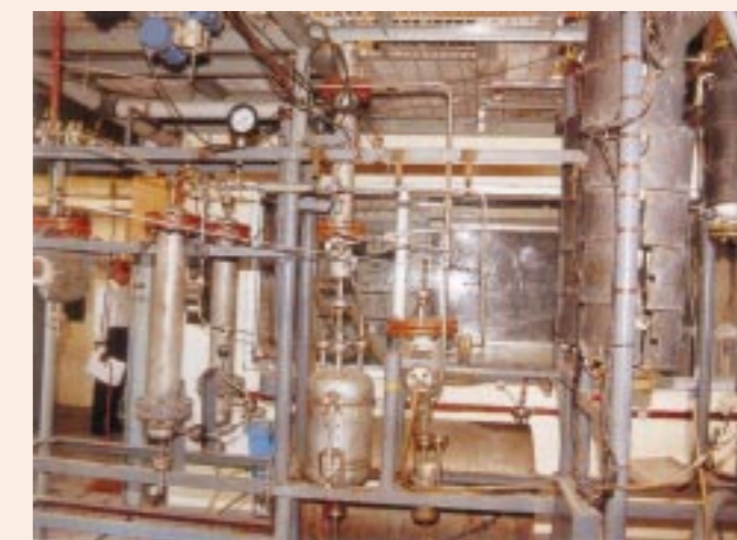
Single tube reactor facility
