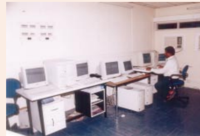
Main Server Room
